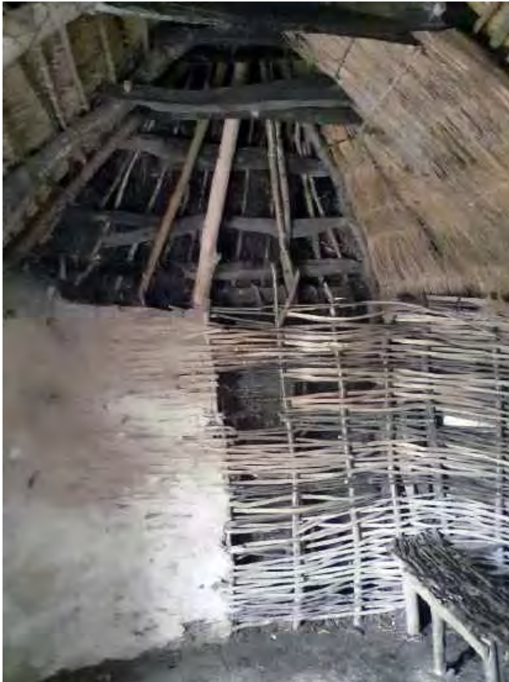
Experimental vernacular construction, National Museum of Ireland (Country Life), Turlough, Co. Mayo (Barry O'Reilly). Such materials and techniques can be traced back to the buildings of our earliest ancestors.
